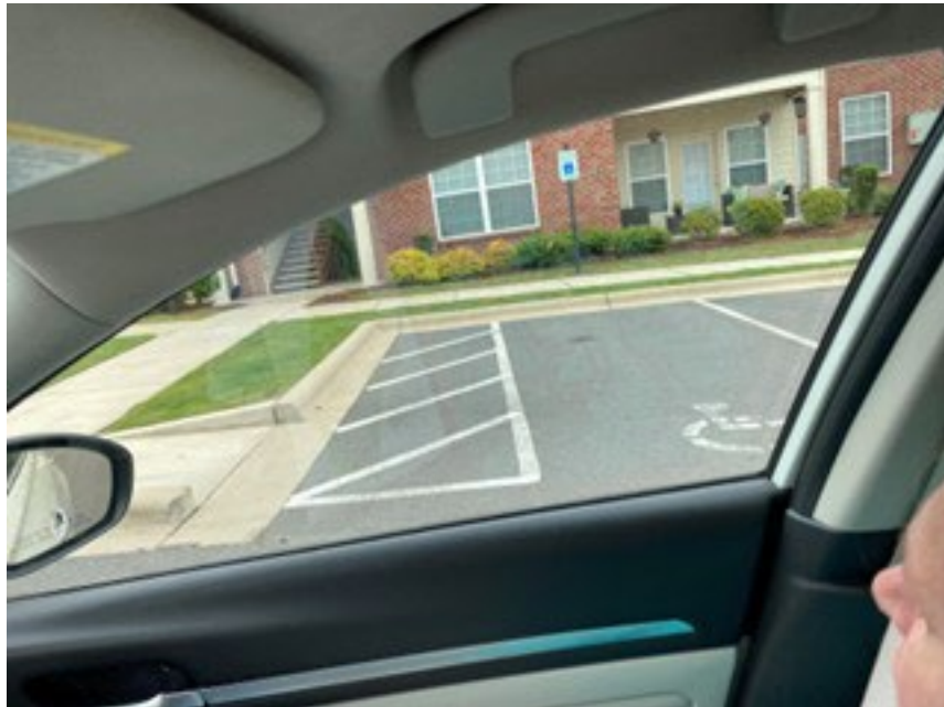
Figure 31: The access aisles for the disabled parking at Revere at Tega Cay are too narrow.
