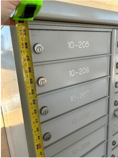
Figure 27: Mailboxes at Revere at River Landing above 48 inches
