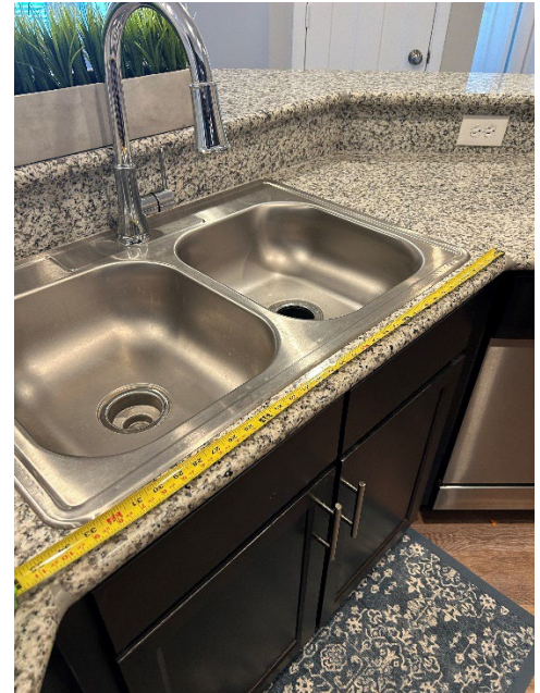
Figure 8: Close-up of kitchen sink in the Craftsman Select floorplan at Revere at River Landing showing lack of clear 30" x 48" inch floor space parallel to the sink.
