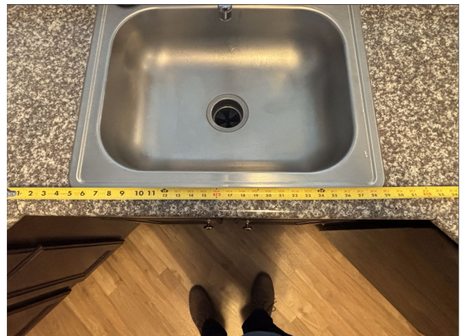
Figure 4: Close-up of kitchen sink in the Craftsman Select floorplan at Worthington Glen showing lack of clear 30” x 48” inch floor space parallel to the sink.
