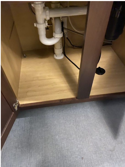
Figure 9: Cabinet structure obstructing knee space under the sink in a bent U shaped kitchen in the Craftsman Select floorplan at Revere at Lake Wylie.
